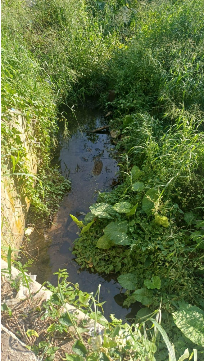
Photo 3a (Taken at C1 Station on 28 May 2026)
